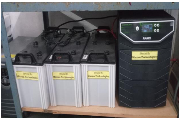
Batteries and Inverters at Kalleda School
